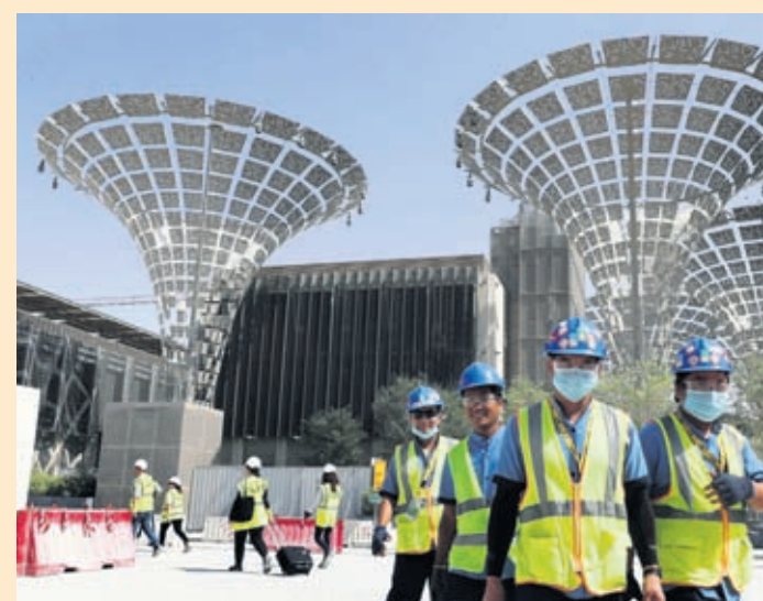
In this Oct. 8, 2019, file photo, technicians walk at the three thematic districts at the under construction site of the Expo 2020 in Dubai, United Arab Emirates.
